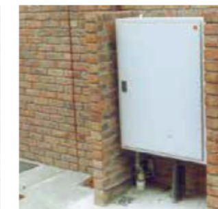
Six meter cabinet
