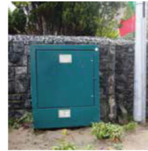
District Regulating Installation (DRI)
