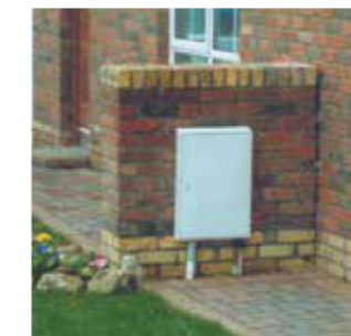
Domestic meter box
